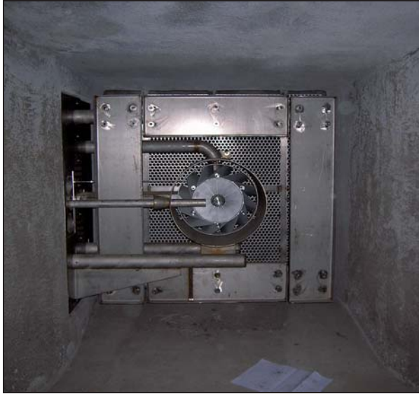
Fig.4 : PILLARD burner type "GRC INDUCT" seen from inside the duct
