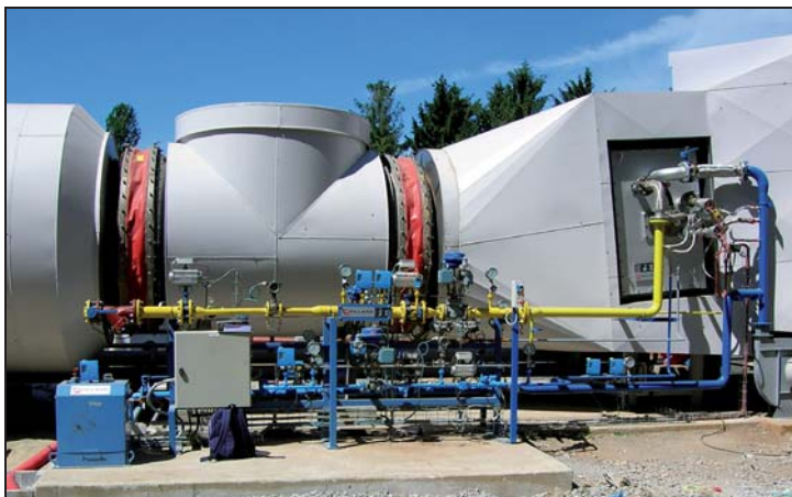
Fig.6 : D.O. pumping set and gas/D.O. valve set
