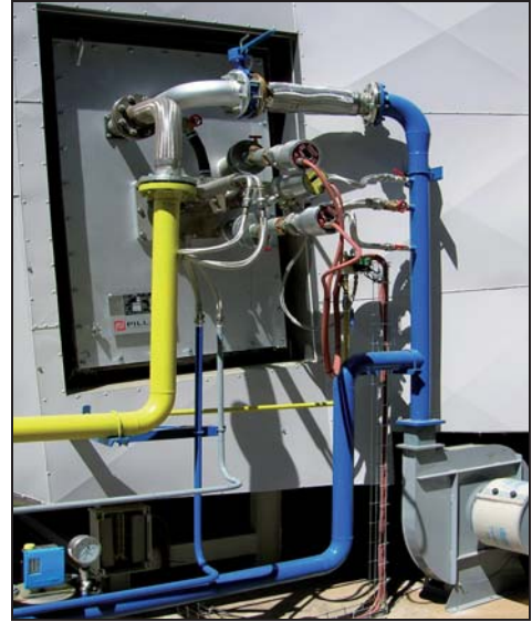
Fig.5 : External view of the burner
