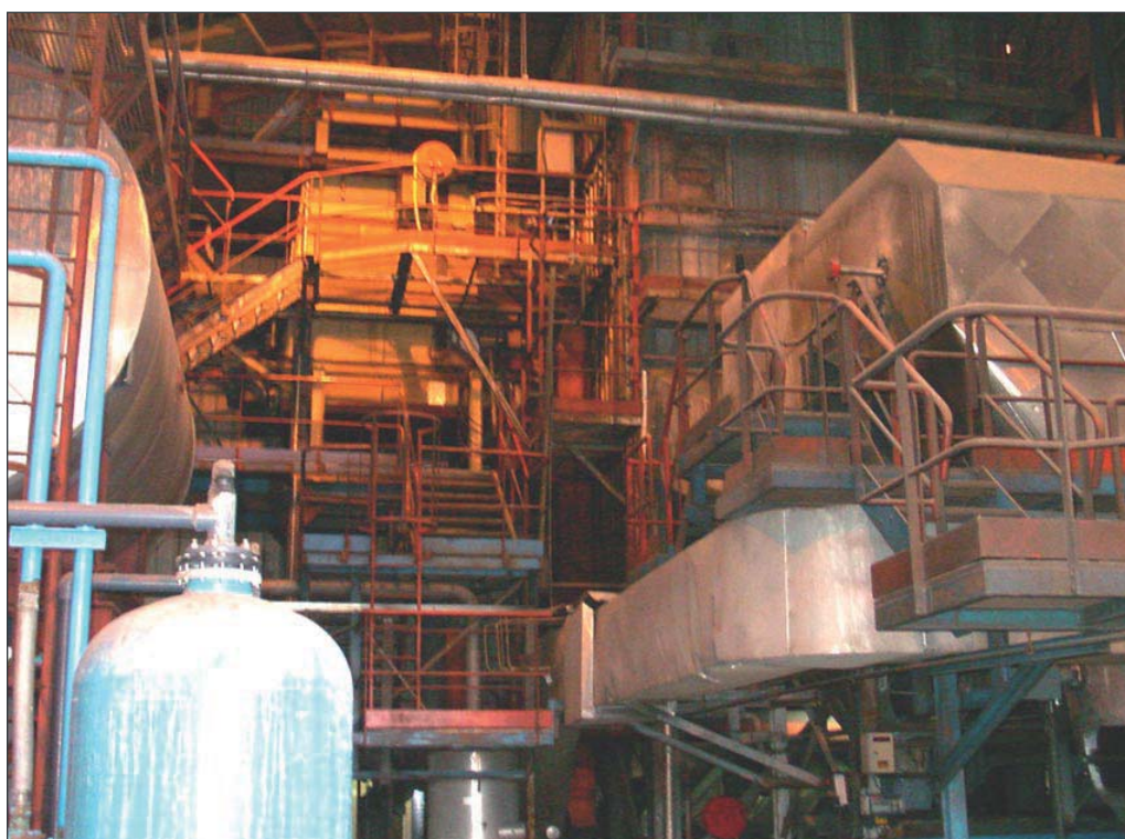
Fig.1: View of the Lardet Babcock 25 t/hr boiler
