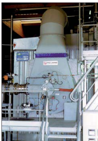
Fig. 2 : PILLARD BIOFLAM® burner fitting one of the three boilers
