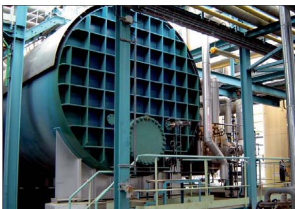
Fig.2 : Reaction furnace - View from the bottom
