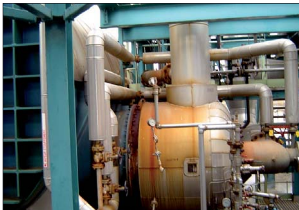
Fig.4 : Acid gas burner tangentially installed on the side of the combustion chamber
