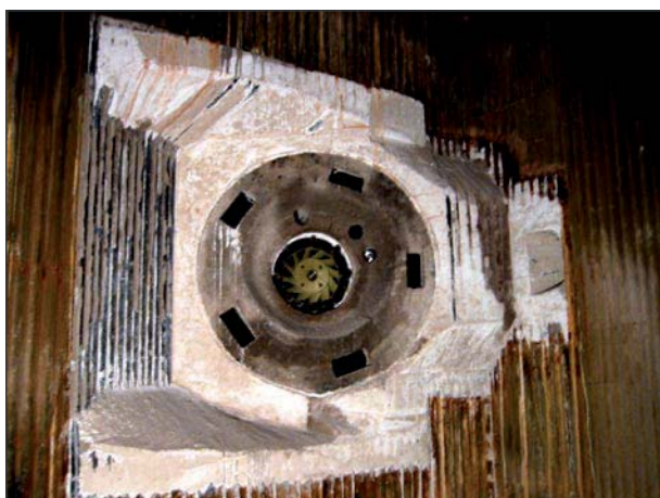
Fig.2 : PILLARD “GRC LONOXFLAM” burner seen from the furnace
