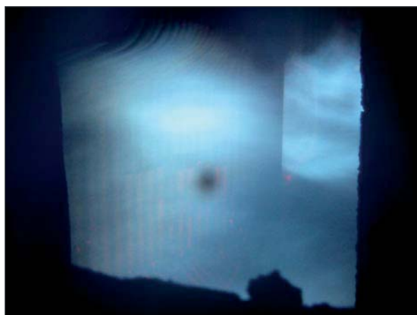
Fig.5 : Flames of the PILLARD “KFT” burners
