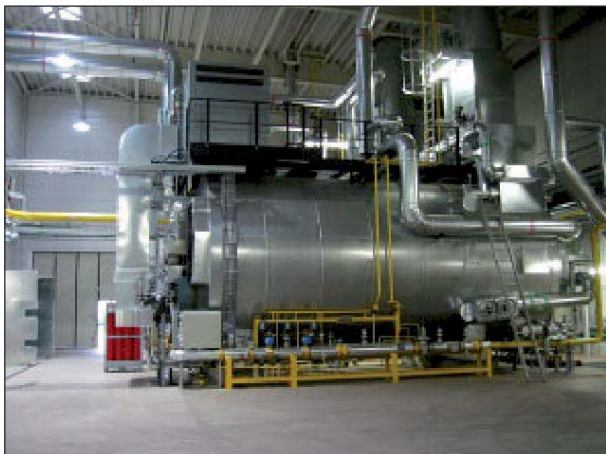
Fig.3 : Boiler n°2 with gas station
