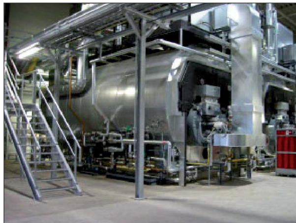
Fig.4 : Boiler n°3 with oil station
