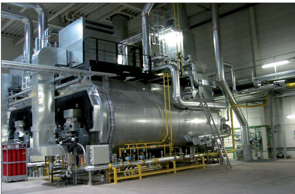
Fig.1 : The two auxiliary boilers
