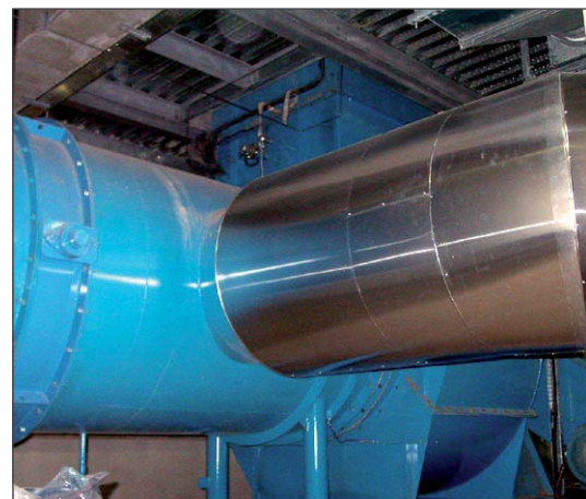
Fig.8 : FGR circuit connected to the combustion air fan inlet
