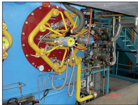
Fig.2 : Partial view of the boiler after upgrading
