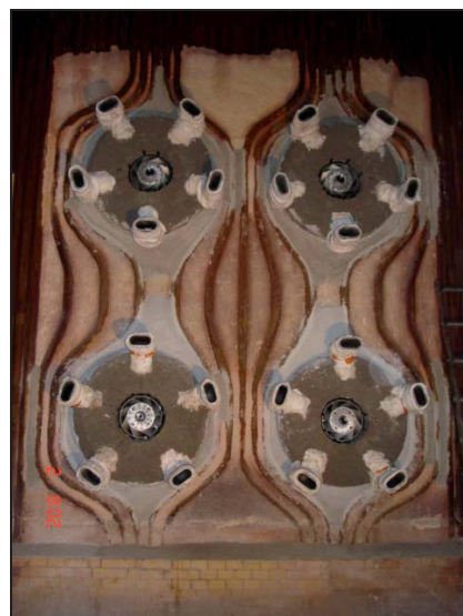
Fig.4 : Inside view of boiler n°2
