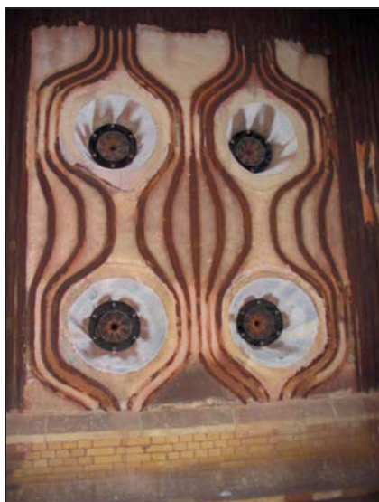
Fig.3 : Inside view of boiler n°2
