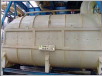
1,300 m 2 reheater - BRAZIL
