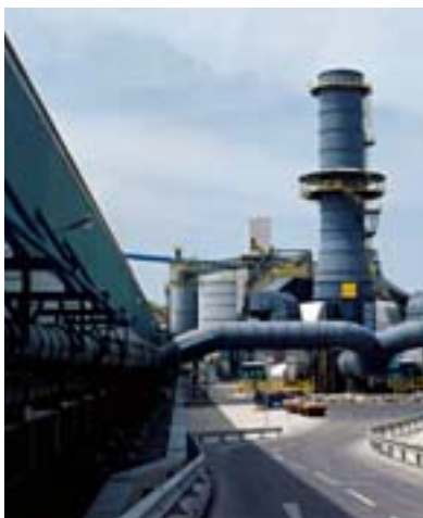
GTC equipped with a Dual Suction System – Alba (Bahrain)
