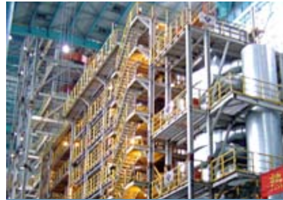
Digiflex® furnace installed by Stein Heurtey on a galvanising line for Ma Steel in P.R. China.
