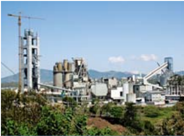
General view of the Holcim cement plant being built in Costa Rica
