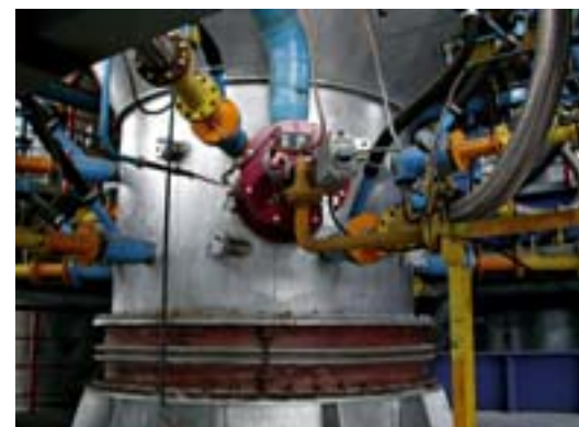
65 MW alumina calciner with 12 injection nozzles for coke oven gas and pilot burner.
